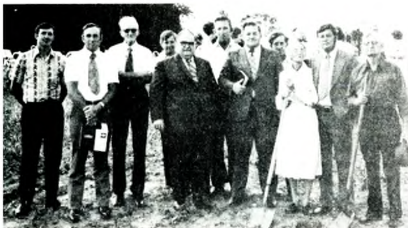
The Monticello (Ky.) First Church recently broke ground for a new facility. Longtime members Georgia Burnett (only living charter member) and Logan Lair turned the shovels of earth. Pictured (l. to r.), back row, are Russell Pyles, Contractor Clyde Carter, Paul Jenkins, Perry Raines, and Charlie Zimmerman; front row—Dempsey Foster, Mayor Carl Shearer, Pastor Eugene Campbell, Georgia Burnett, Curtis Bell, and Logan Lair.
